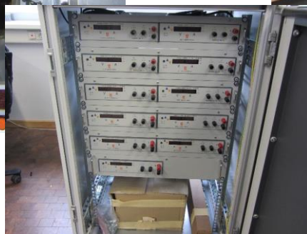
power supplies for control
