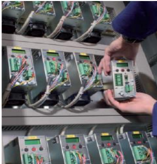
G-ELI Facility management- Instrumentation - Process control
